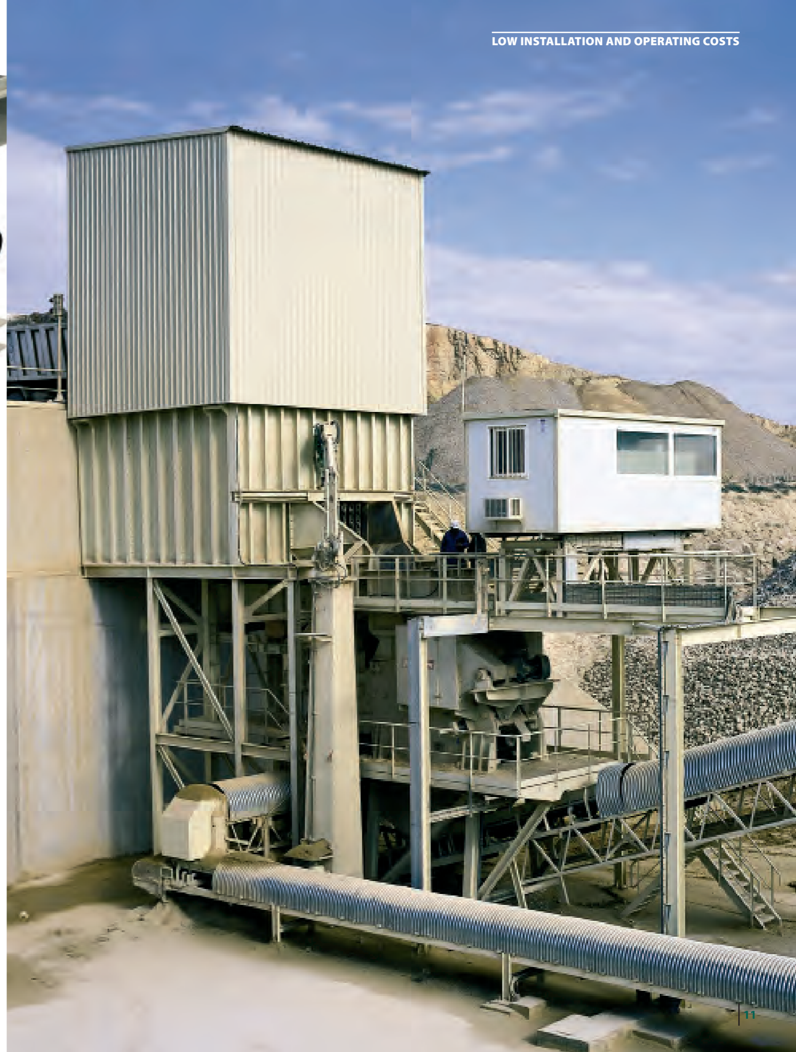
A Nordberg C140 jaw crusher in a stationary installation.
