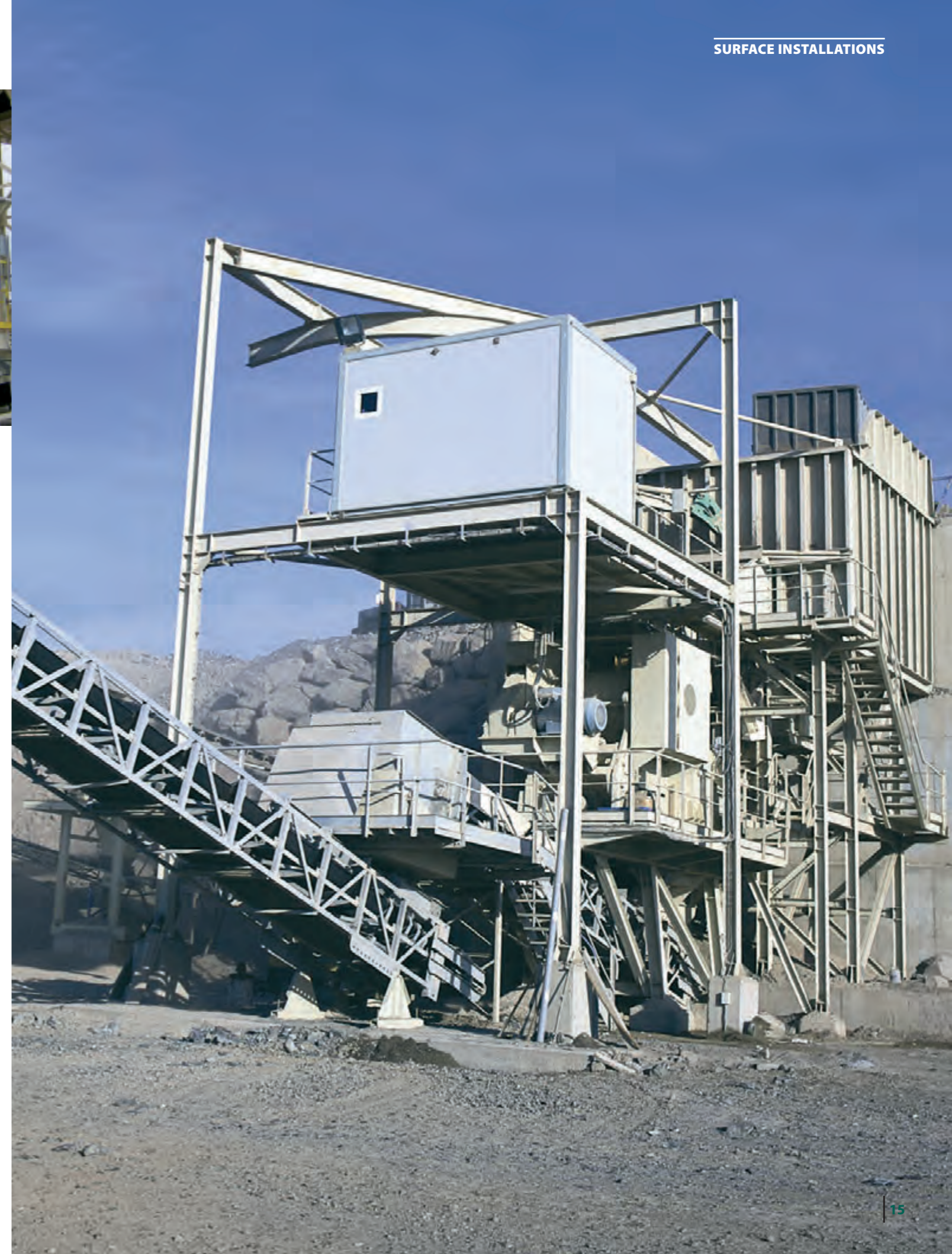
A Nordberg C145 jaw crusher in a stationary installation.
