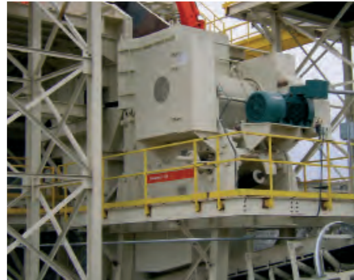
A C145 during the installation phase at a new primary crushing plant.
