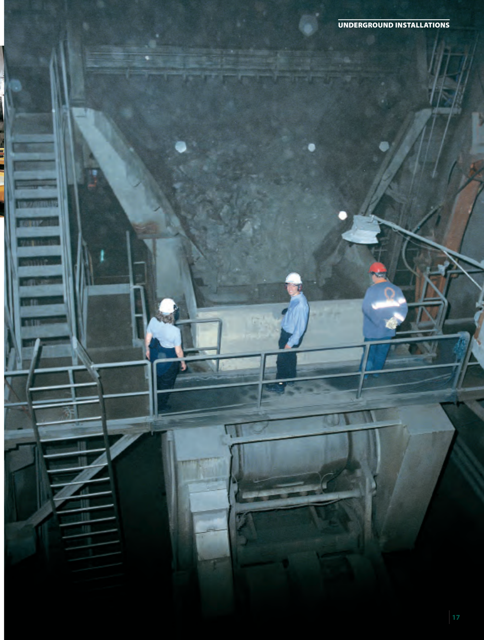
C200 in operation in a zinc and copper underground mine 1400 meters below ground. The crusher is monitored and operated from the surface control room.
